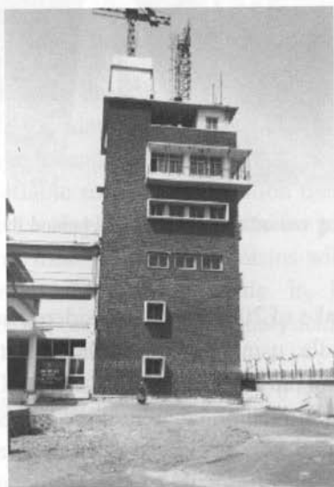
Fig. 1.18 A view of the tilted HMT building.
