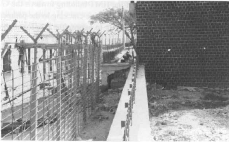
Fig. 1.20 Lateral spreading caused the parapet walls behind the HMT building to crack severely.
