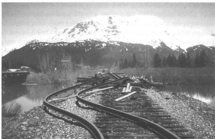
Fig. 4.1 Damage to a railway embankment during the 1964 Alaska earthquake due to lateral spreading of a river valley. (Photo from USGS).
