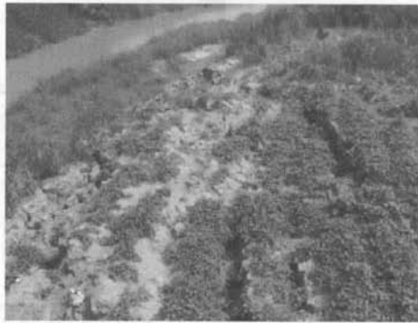
Fig. 1.15 Lateral spreading next to a river channel during the 921 Ji-Ji earthquake, Taiwan.
