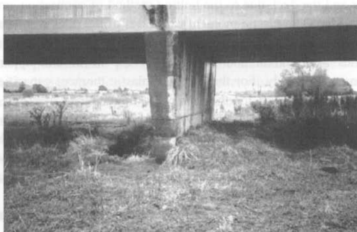
Fig. 1.13 A view of Pier C in laterally spreading soil.
