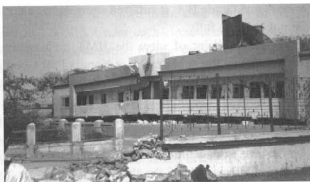
Fig. 1.19 A view of the collapsed two-storey building.
