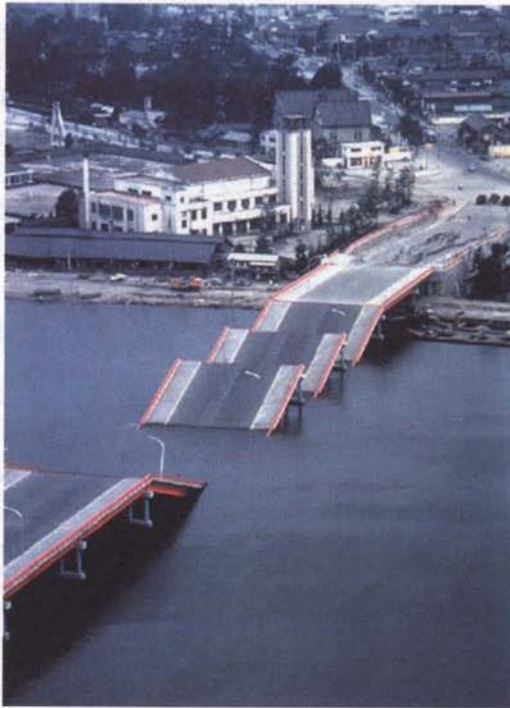
Fig. 1.5 A view of the collapsed Showa bridge (Photo by V V Bertero) Courtesy of National Information Service for Earthquake Engineering EERC, University of California, Berkeley.
