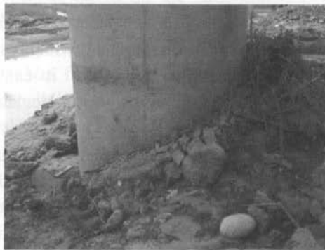
Fig. 1.16 Passive bulge and gap formation next to a bridge pier following lateral spreading.
